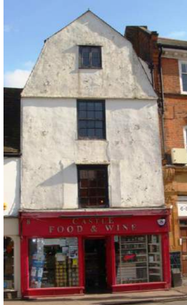
Picture 46. Upper floors to No. 8 The Wash in need of refurbishment.
