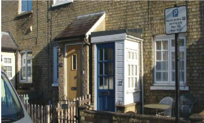
Picture 98. Inappropriate porch detailing.
